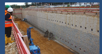
These walls will be diaphragm walls or "D-Walls" for short. They are built deep into the ground in solid concrete rectangular sections which are interlocked with watertight vertical joints. Horizontal rods called tiebacks help stabilize these walls.
